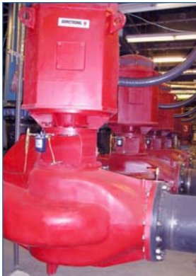
Enwave District Cooling Facility, Toronto, Canada.
