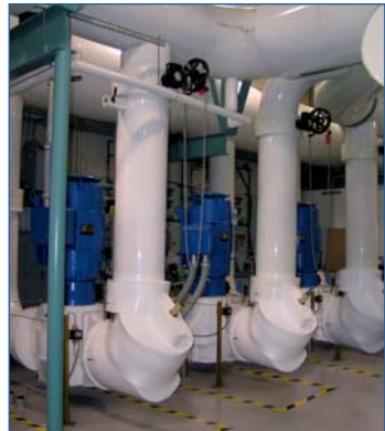
District Cooling Project, Phoenix, U.S.A.
